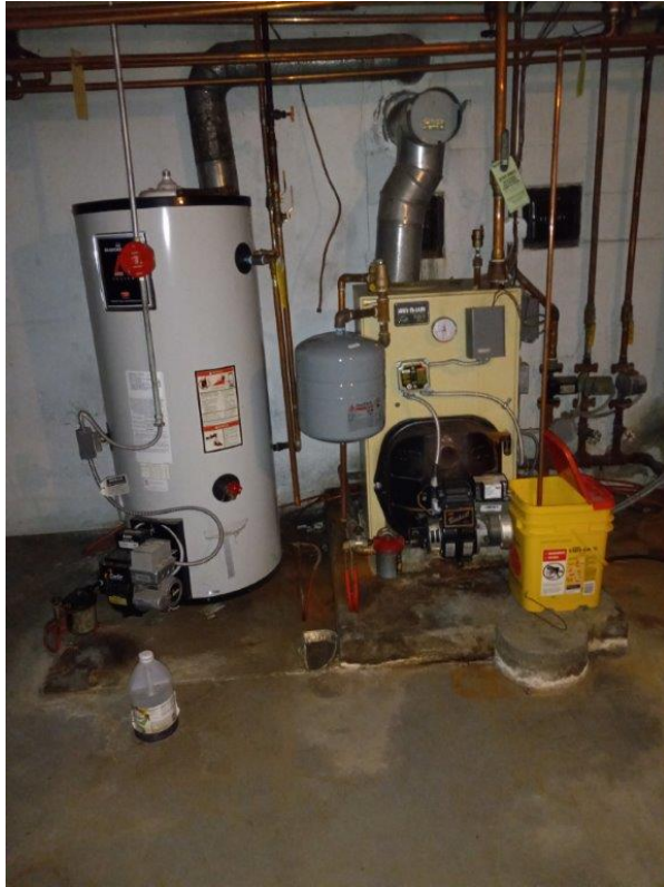
Oil furnace and water heater
