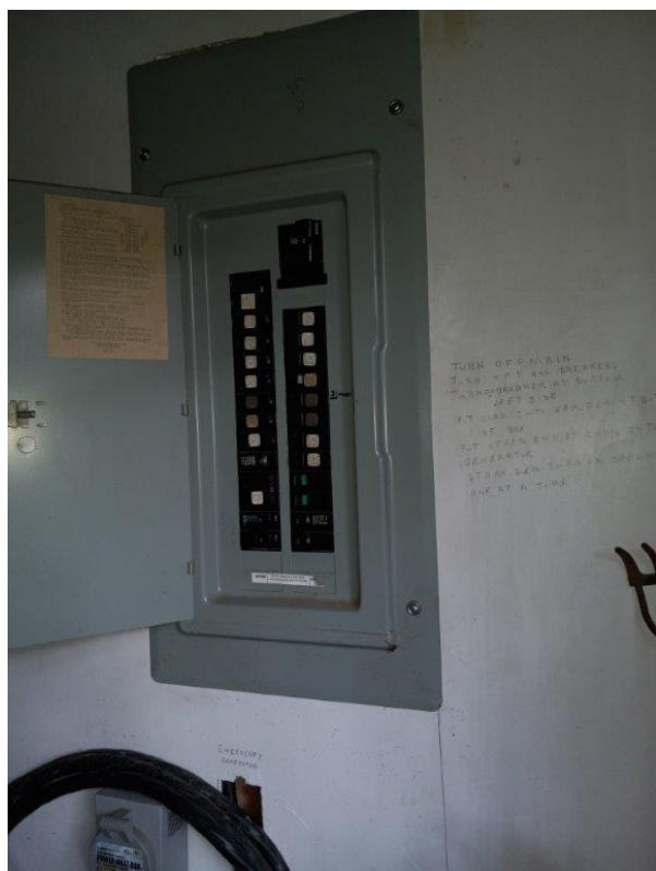
Garage panel with generator hook-up
